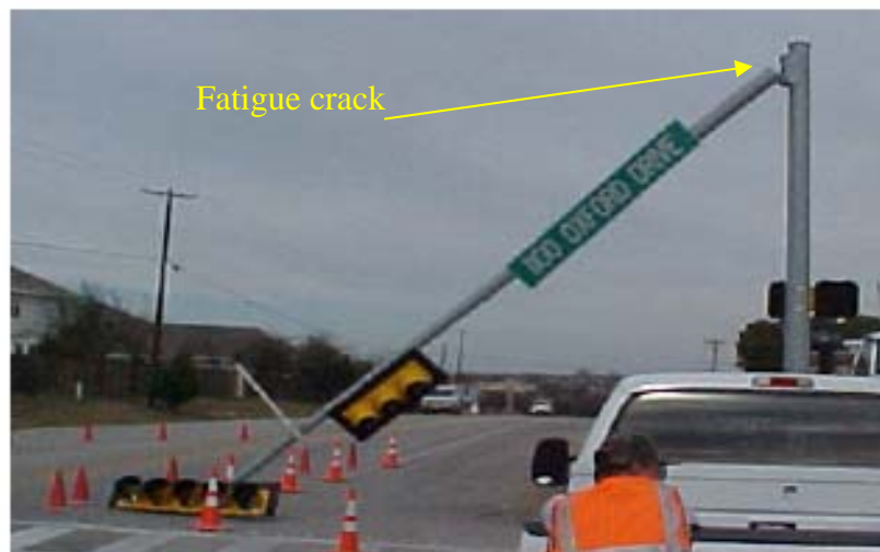
Figure 1.2 Traffic signal structure failure in Pflugerville [11]
